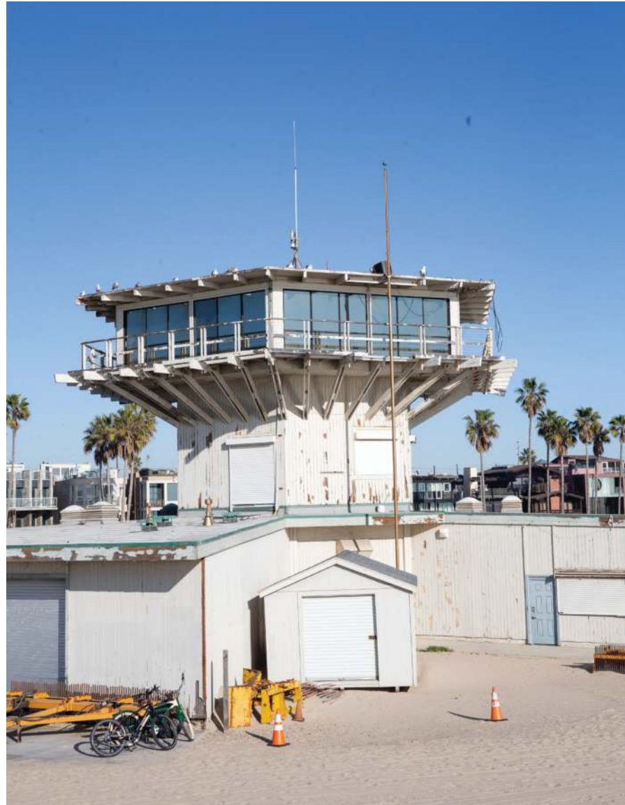
The Venice Lifeguard Station's current appearance is dilapidated, with paint coming off the exterior and construction equipment surrounding the building.
